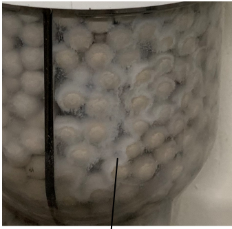
Figure 9: Salt precipitate deposited on neutralization media from Aluminum heat exchangers
